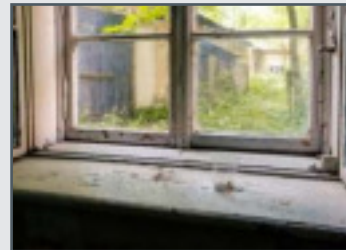
Window, Wall and Floor Damage
