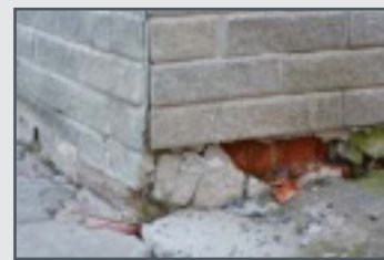
Foundation Damage & Basement Flooding
